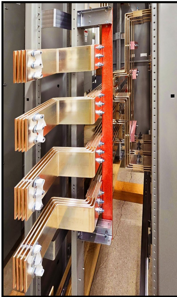
Figure 18: Building 48 Denver Federal Center Electrical Denver, CO
