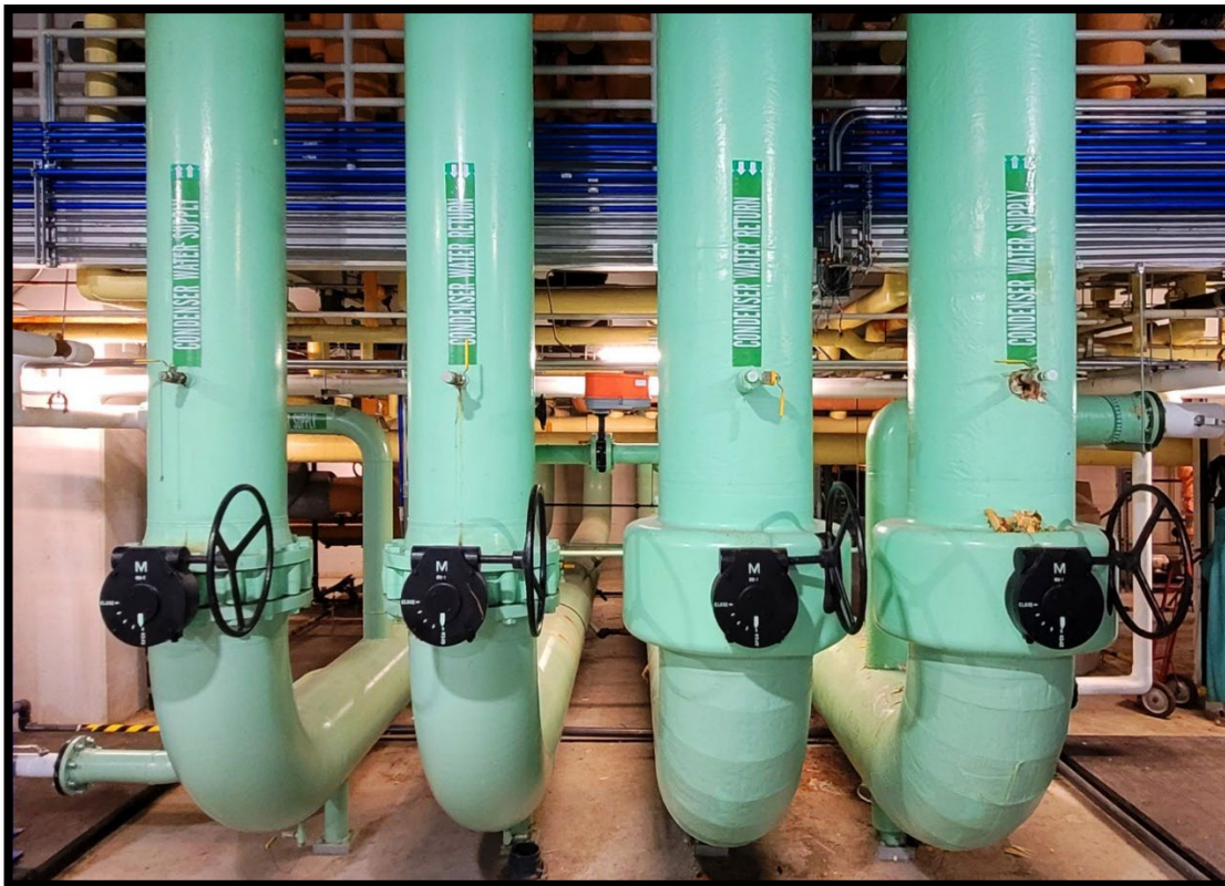
Figure 16: Ronald Reagan Federal Building Mechanical Piping Washington, DC
